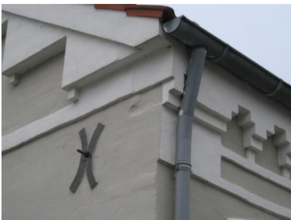
Slotsgade 14 - blokgesims, muranker
